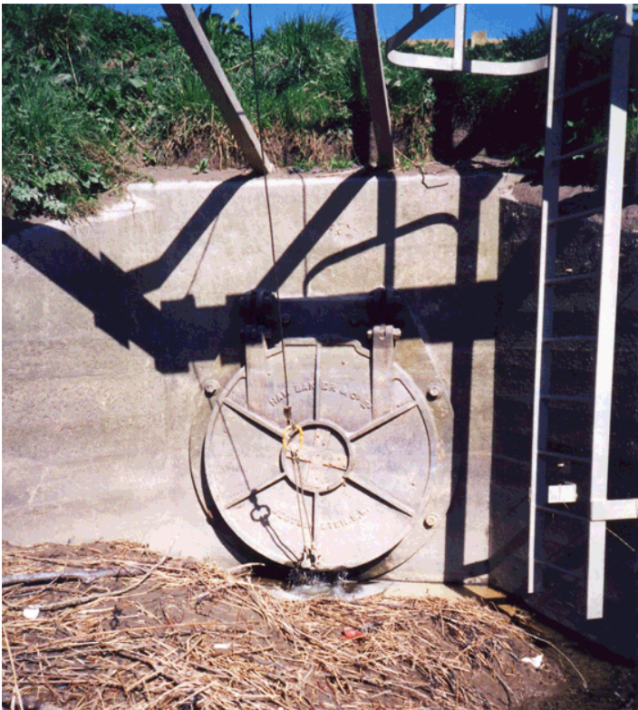
Figure 6. Tidal flap gate on the Severn.
